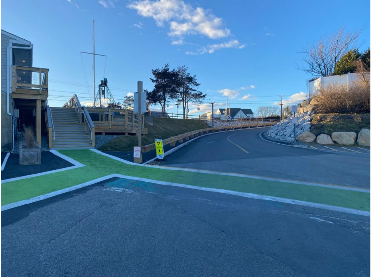
New Deck and Stairs at Wharfinger Building. New sidewalk along Barcliff Ave. Ext.
